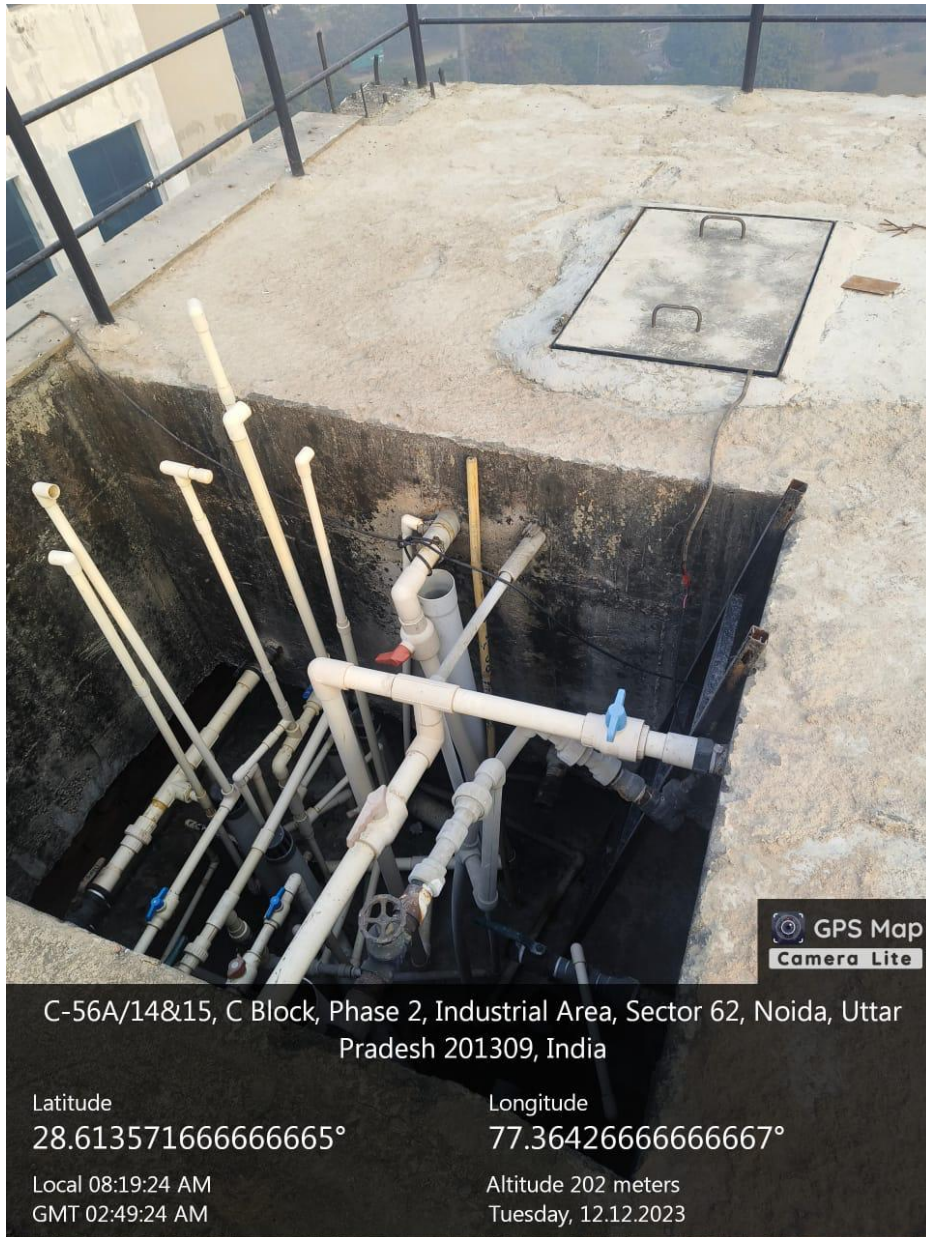
Water Drainage system at the basement area
